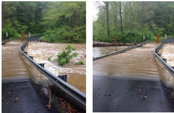
Figure 1. Flooding at Swift Run Bridge, Albemarle County in 2017
